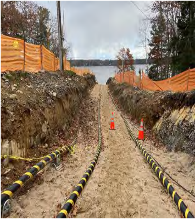
Fig 1: Cable trench on the Getchell property/west side of the Bay. Viewing east. (11-08-19).
