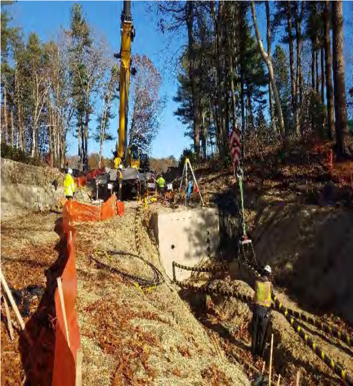
Fig 13: Pulling cable into the vault at Gundalow landing/east side of the Bay. Viewing east. (11-13-19).
