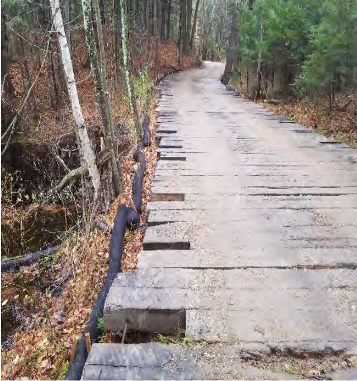
Fig 9: Filter sock installed on access road off of Route 4. Viewing east. DW 204. (11-12-19).
