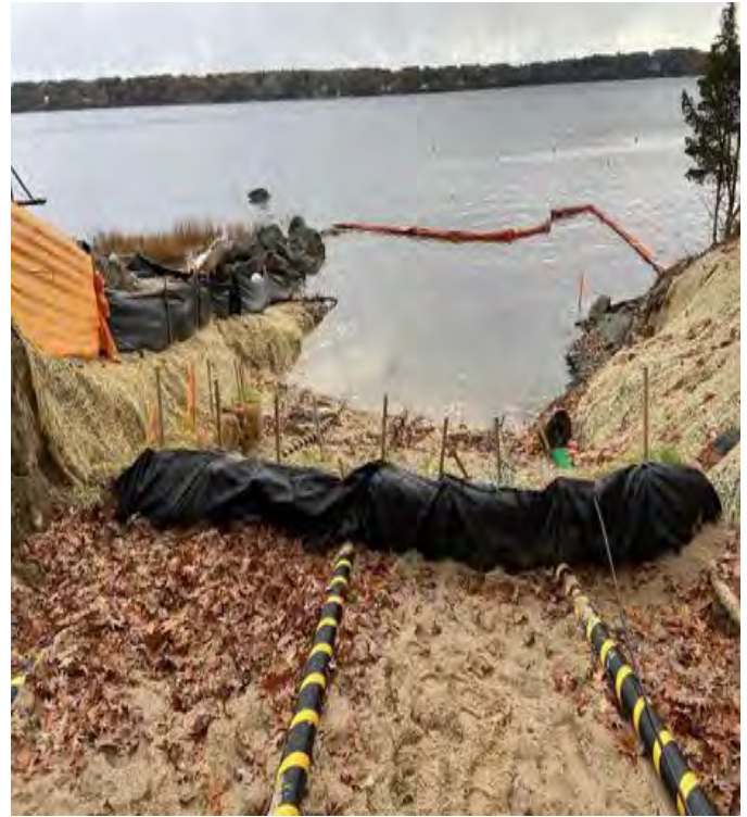
Fig 2: Sediment controls installed in cable trench at Getchell property/ West side of the Bay. Viewing east. (11-08-19).
